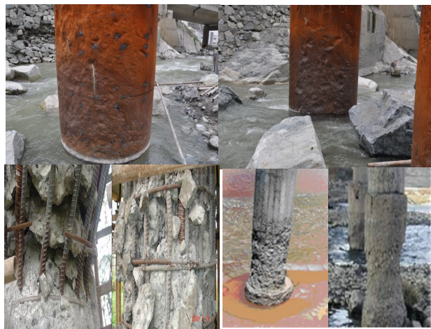
图1 映卧公路青岗坪鱼子溪大桥桥墩遭受泥石流冲击破坏 Fig.1 Damage of bridge pier by the impact of debris flow at Yuzixi, Qingpinggang, Yingwo highway
